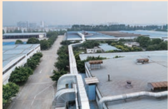
• Air Pipes for VOCs Tail Gas Treatment Project of Container Coating Line
