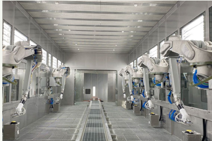
Ji'nan Commercial Vehicle Company built water-based paint coating lines
