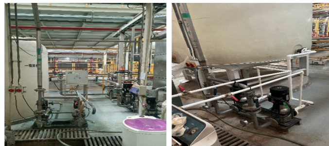
Project of reusing concentrated water from coating by Ji'nan Light Truck Company
