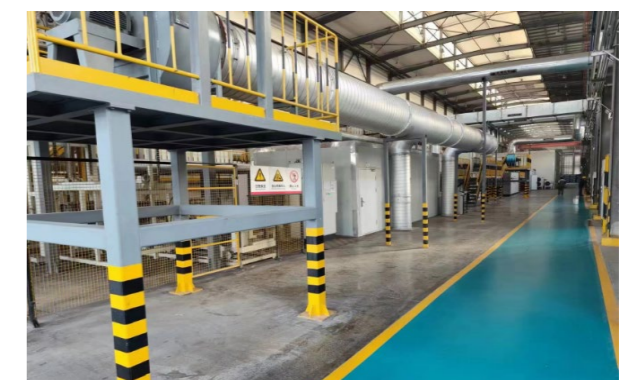
Technical transformation project of Ji'nan Molding Plant for a more intelligent and environment-friendly casting coating line
